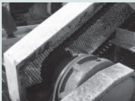
✗ Chain drive not fully guarded
