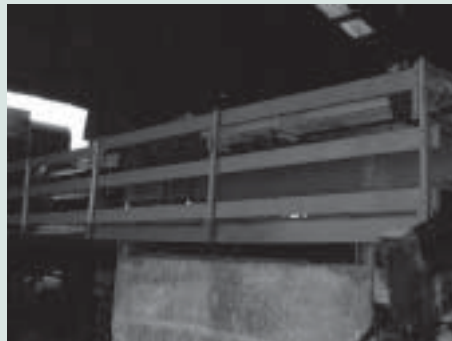
✔ Handrails must be solidly built with mid rail and, where needed, kickboard
